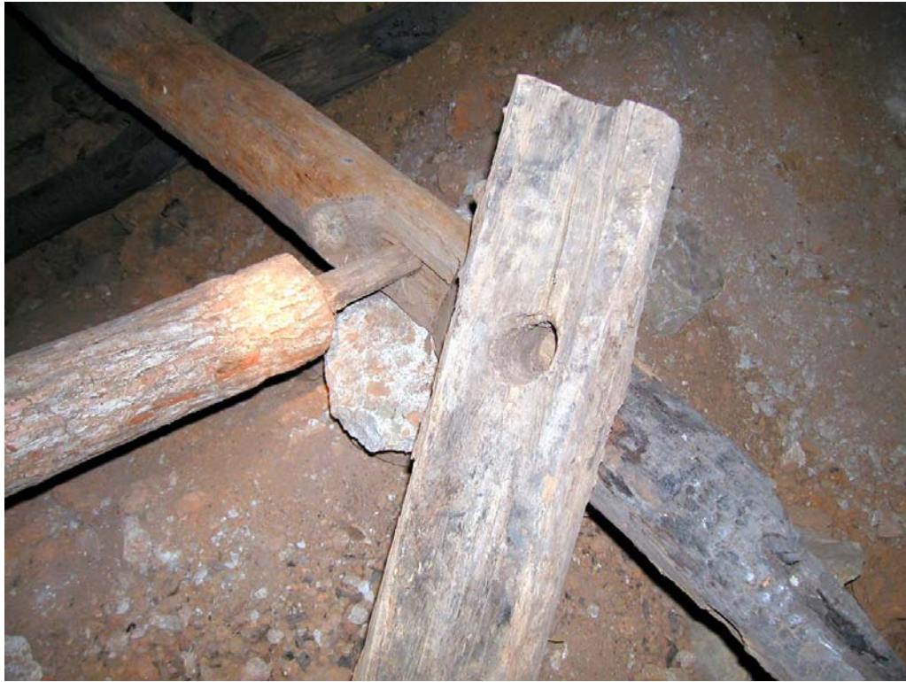
Figure 20. Mortise-and-tenon joint used to secure the frame corners of the leaching vats in Cagle Saltpetre Cave.
